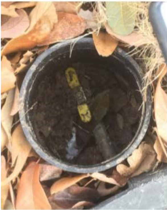
Exterior Water Cutoff (turned on)
