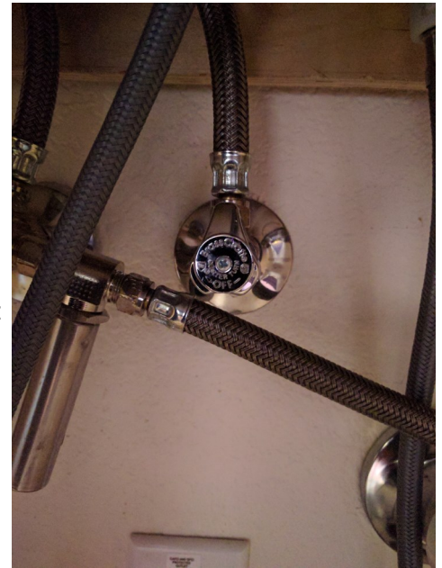
Example of cut-off valve underneath a sink.
