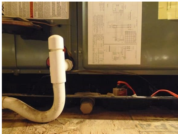
Condensate Line located at air handler
