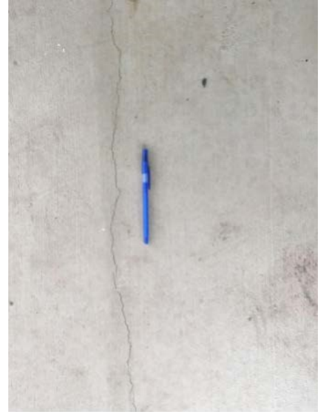
A normal sized crack in concrete
