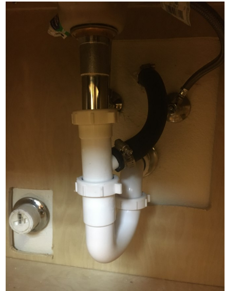
The black pipe is your primary condensate line
