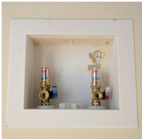
The plumbing for your laundry washing machine. The drain goes into the capped porting in the center of the two water spigots.
