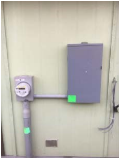
Your Exterior Circuit Breaker panel is near the electrical meter
