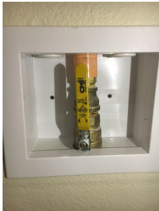
Interior Water Cutoff (turned on)
